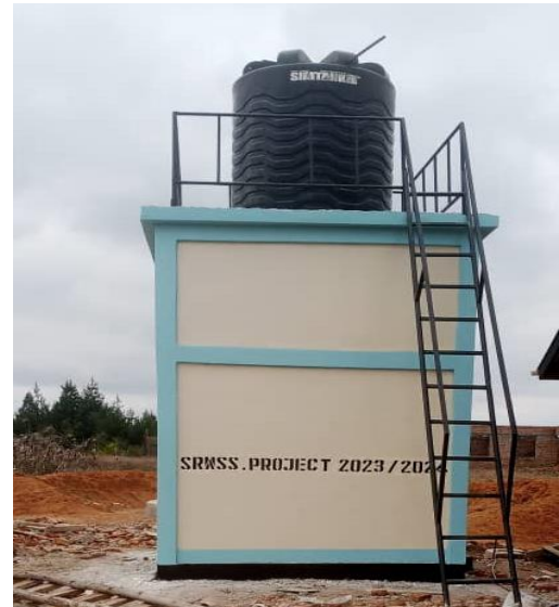
Elevated water tanks at Masege Dispensary, Kilolo D.C, Iringa Region
