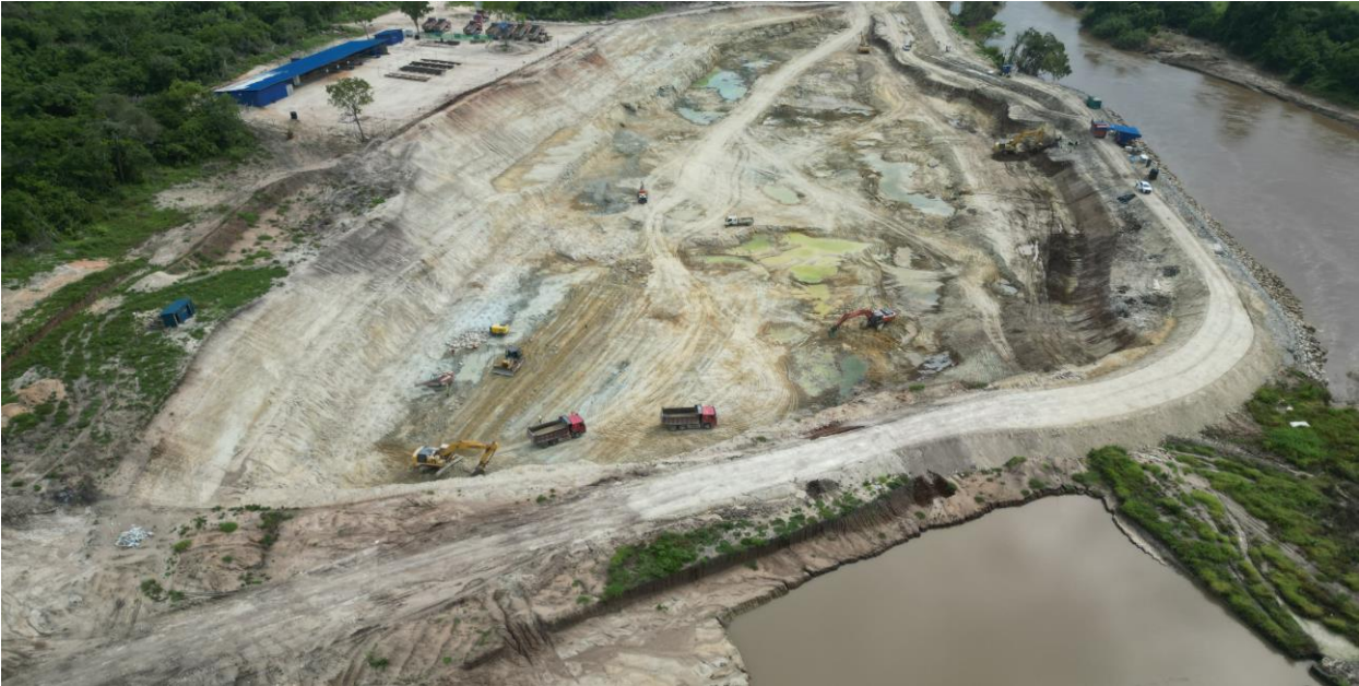
Construction of the Kidunda Dam Project along the Ruvu River, WamiRuvu Basin, Morogoro Region
