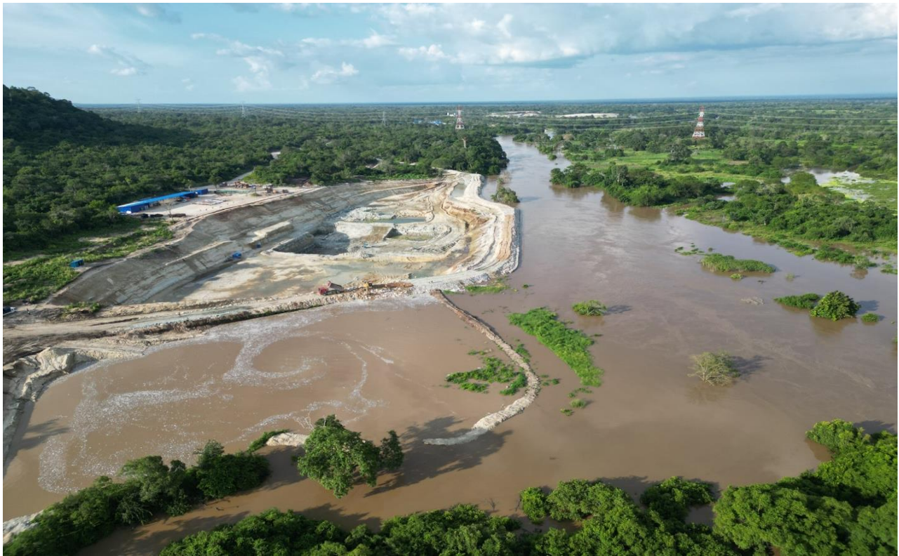
Construction of the Kidunda Dam Project along the Ruvu River, WamiRuvu Basin, Morogoro Region
