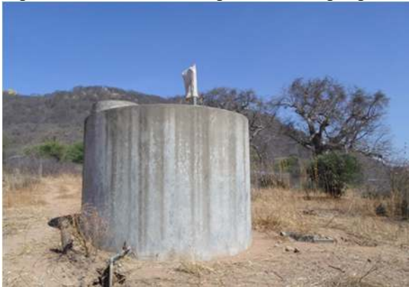
Figure 5.5: Water tank at Bubutole
