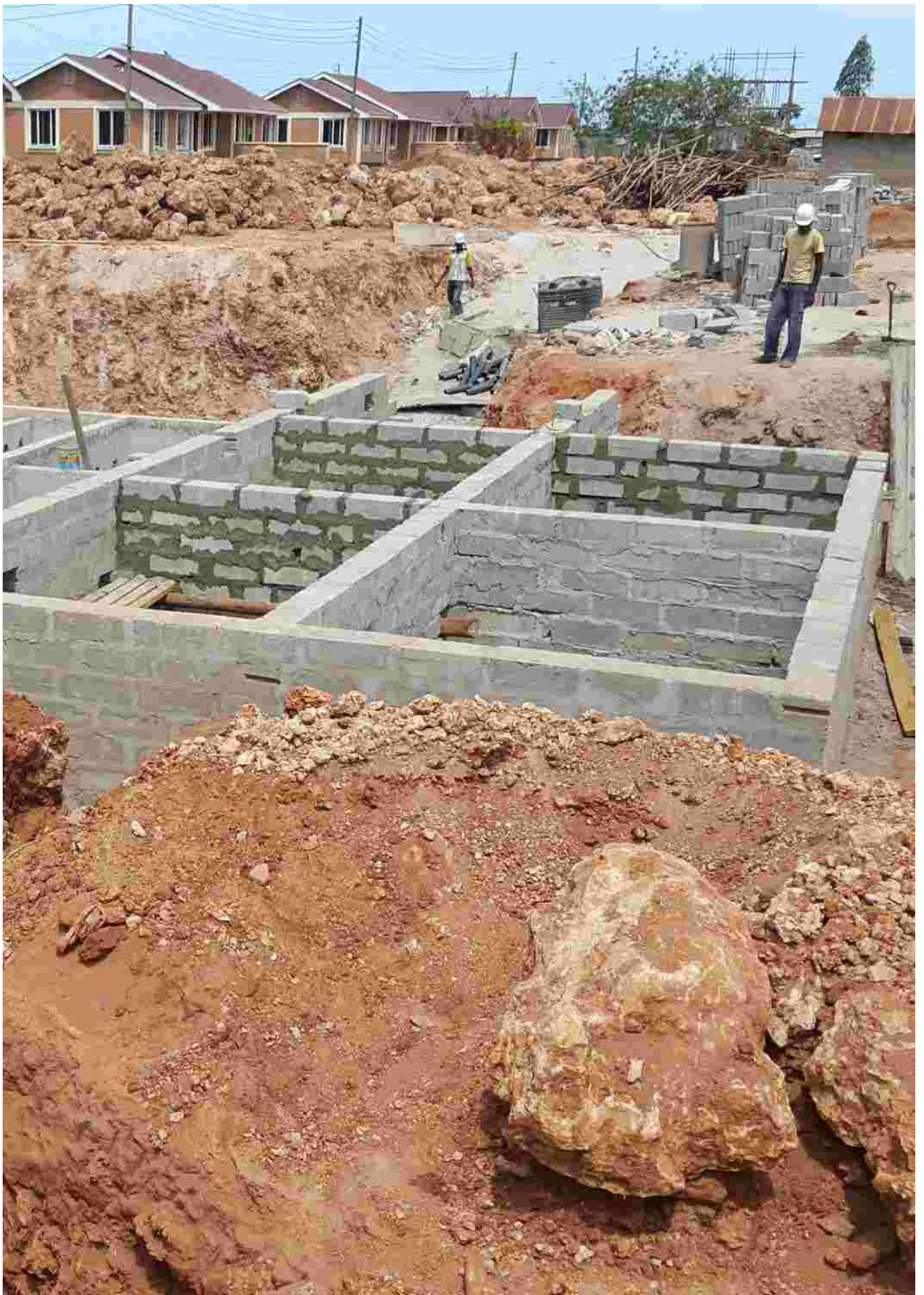
National Housing Corporation (NHC) Mwongozo Affordable Housing Development, Kigamboni, Dar es Salaam On-site wastewater management system (designed by BORDA Tanzania) with septic tanks, simplified sewers, ABR, AF, PGF and sub-surface water distribution network.
