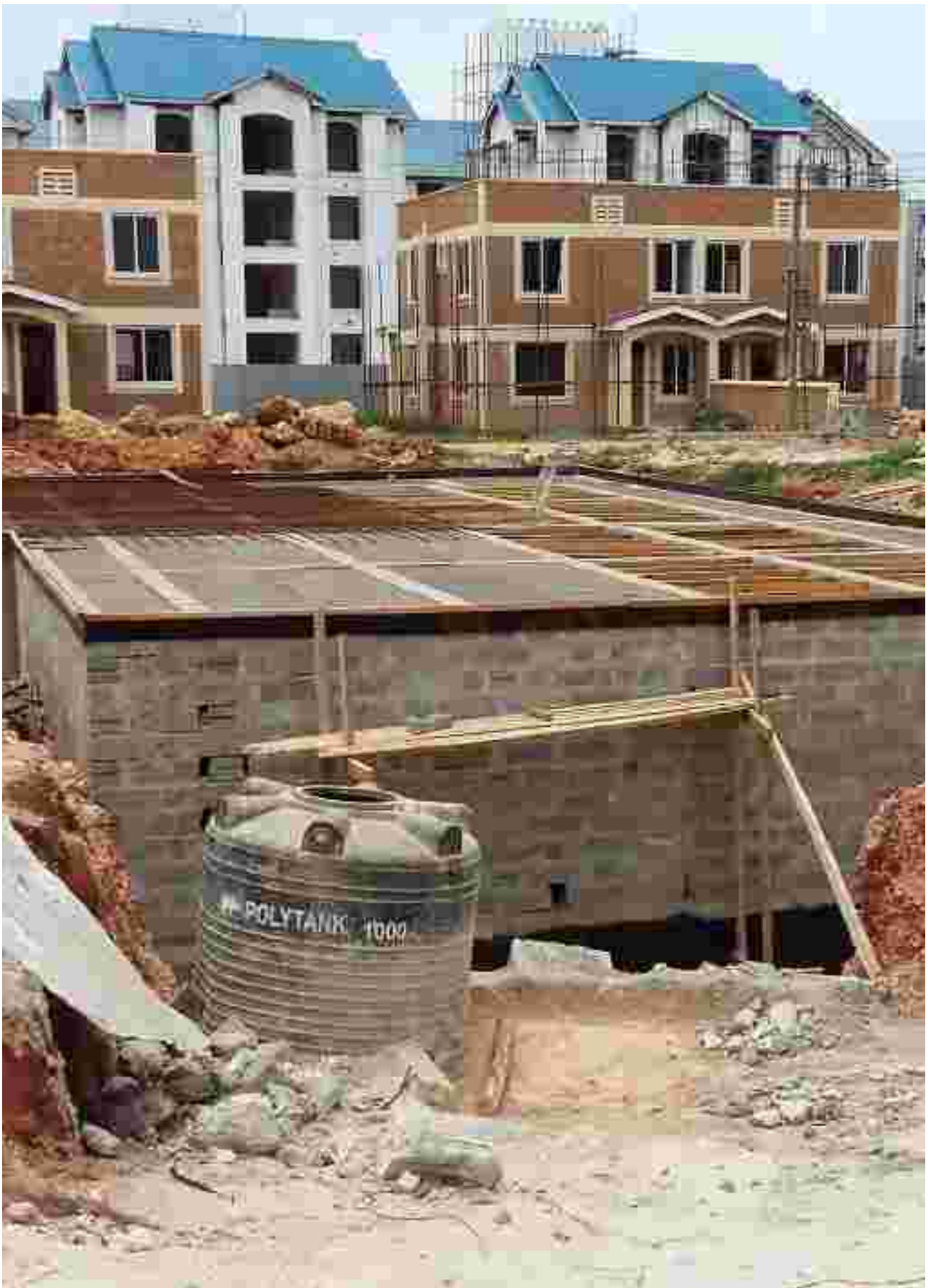
National Housing Corporation (NHC) Mwongozo Affordable Housing Development, Kigamboni, Dar es Salaam On-site wastewater management system (designed by BORDA Tanzania) with septic tanks, simplified sewers, ABR, AF, PGF and sub-surface water distribution network.
