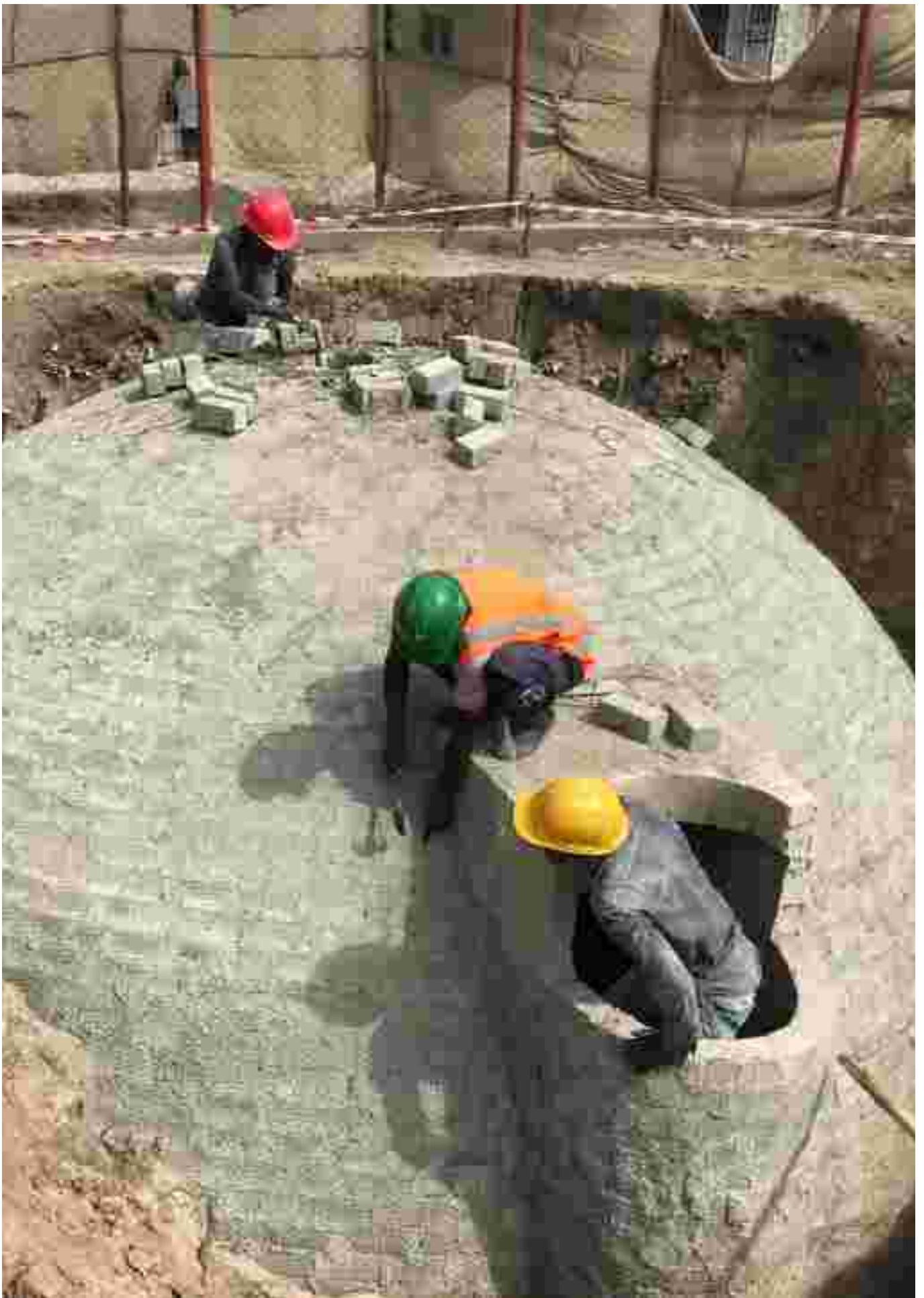
Faecal Sludge Treatment Plant, Mburahati, Dar es Salaam. Faecal Sludge Treatment Plant (designed by BORDA Tanzania, financed by UKAID) with Biogas Settler, ABR, AF and sub-surface water distribution system. The FSTP produces biogas for cooking purposes, and treated wastewater is used to irrigate the surrounding vegetation.
