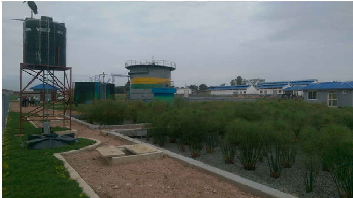
Photo: Wastewater treatment facility of abattoir (bio digester)
