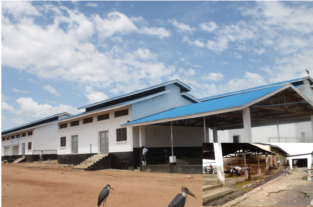
Photo: Rehabilitated Mwanza City abattoir. The small photo at the right bottom corner is the abattoir before rehabilitation
